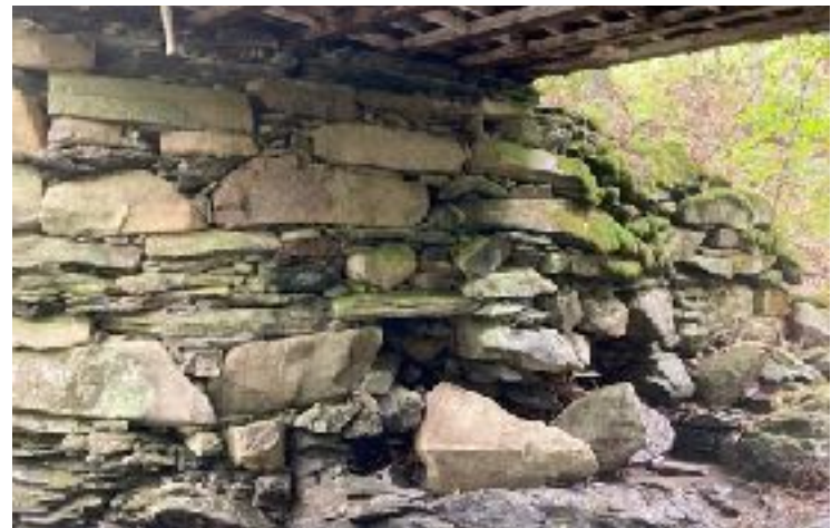
Figure 2 Abutment starting to collapse
